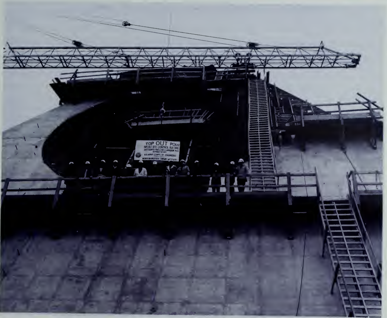
Fig. 2-27. Despite weather conditions, which ranged from -40^{\circ}\text{F} to 100^{\circ}\text{F} , the Top-Out Pour for the Missile Site Control Building took place on 12 October 1971.
